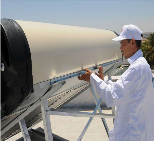
Tank centered and horizontal position
