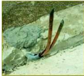
Figure 11: New SWH connection have to take into account existing piping
