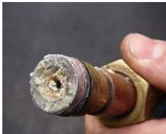
Figure 33: Pipe clogged with limestone
