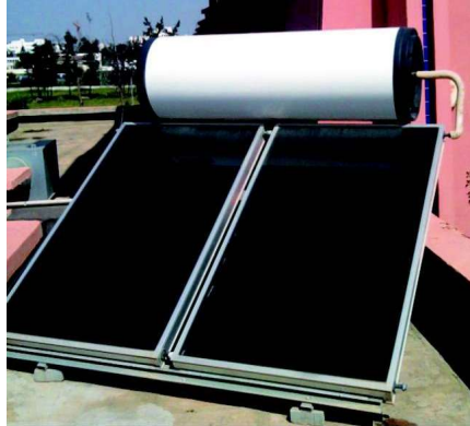
Figure 8: Individual Solar Water heater
