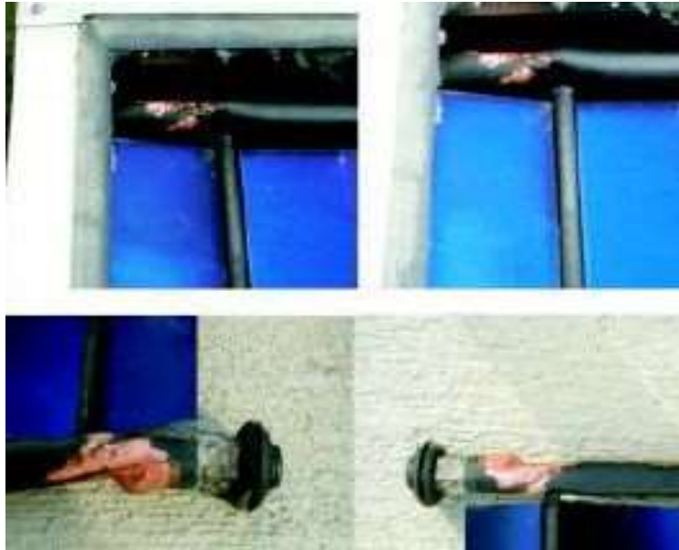
Figure 34: Pipe bent due to incorrect tightening
