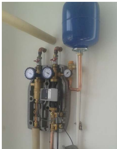
Figure 25: Expansion tank location close to the pump station
