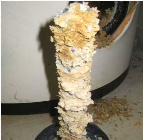
Magnesium anode control and replacement
