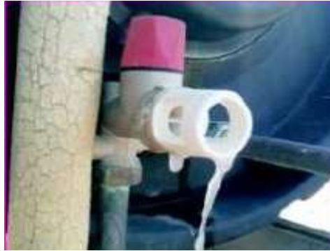
Figure 36: Safety group leaking
