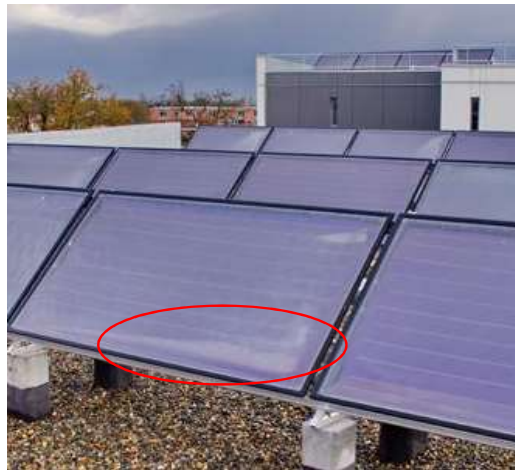
Figure 30: Condensation holes under the glass
