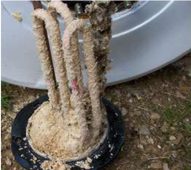
Electrical resistance control and replacement
