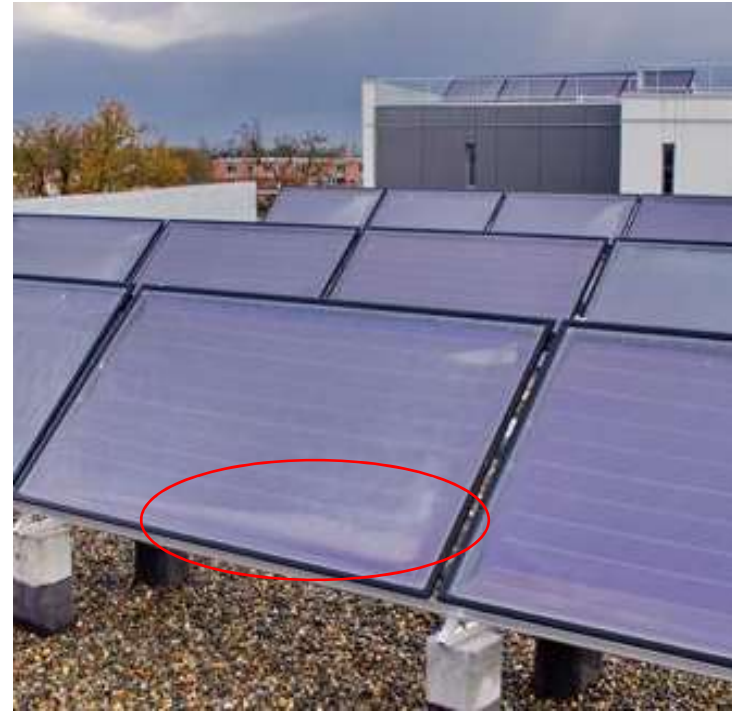
Condensation holes under the glass
